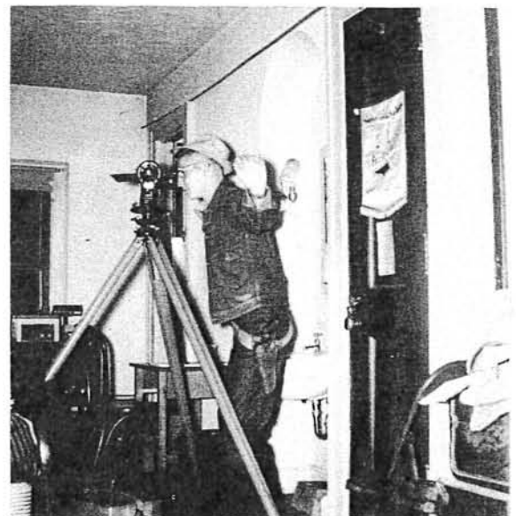
The railroad's coming through the middle of the house
